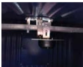
Dingtek DF702 instalado num Cyclea
